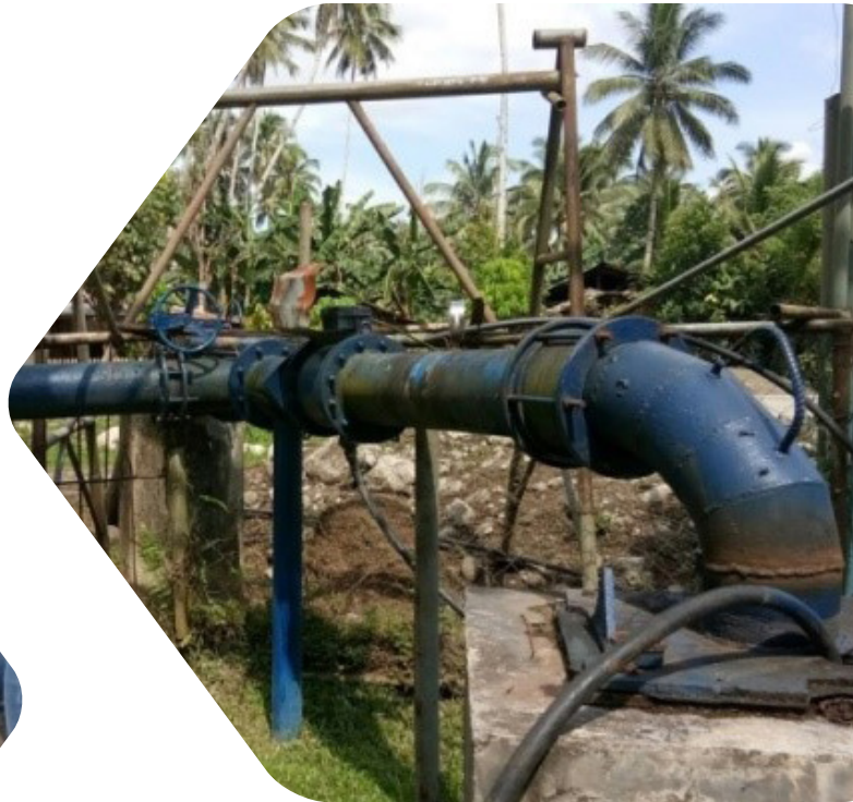
Pump Station No.17
