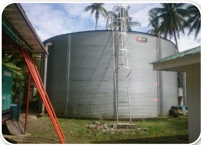
KM 6, LIBERTAD Ground Reservoir and Booster Station
