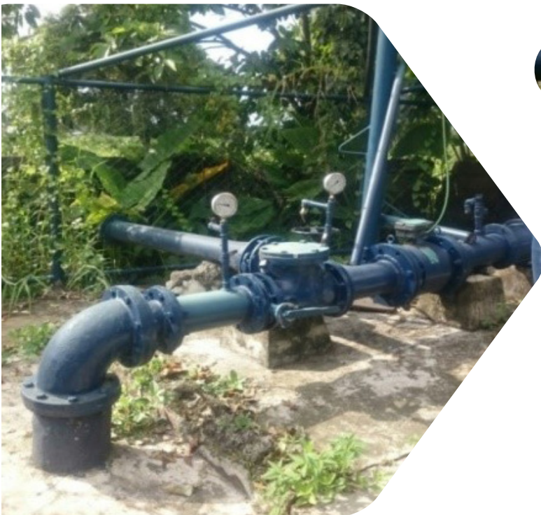
Pump Station No.03
