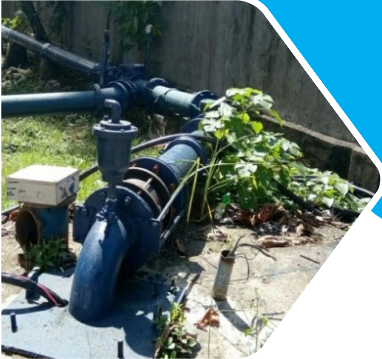
Pump Station No.01
